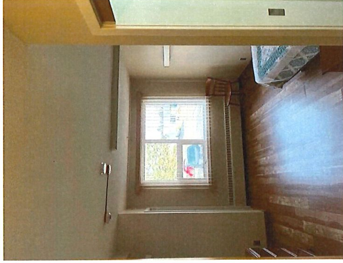
Minimum building standards not met
